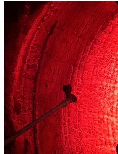
Applied on the walls of Ladle & Furnace
